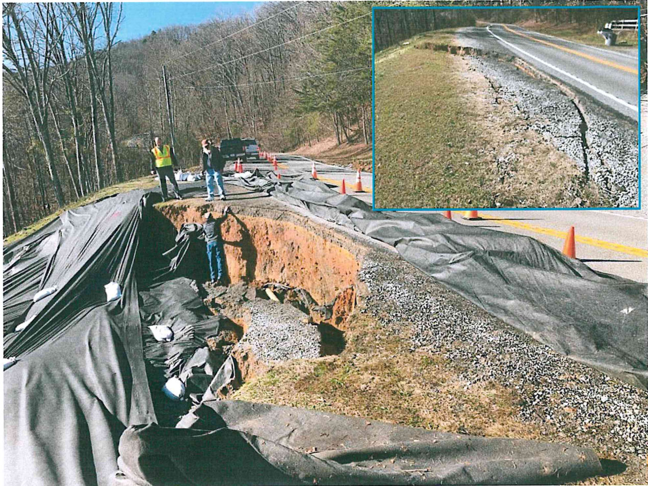
Photo 1: Landslide extending from edge of pavement to toe of slope at private driveway
